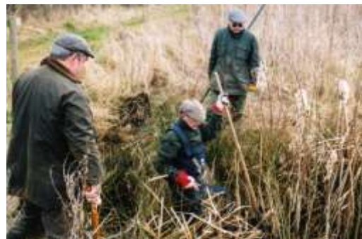
Clearing a culvert to regulate water levels - Work parties are an essential management tool.. PMJS
